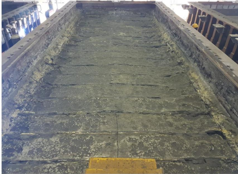
Figure 15. Cathode surface of the first full copper collector bar pot at the age of 1002 days.
